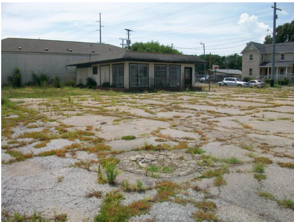
Photograph 4 – View of the depression in the asphalt located on the eastern portion of the subject property.
