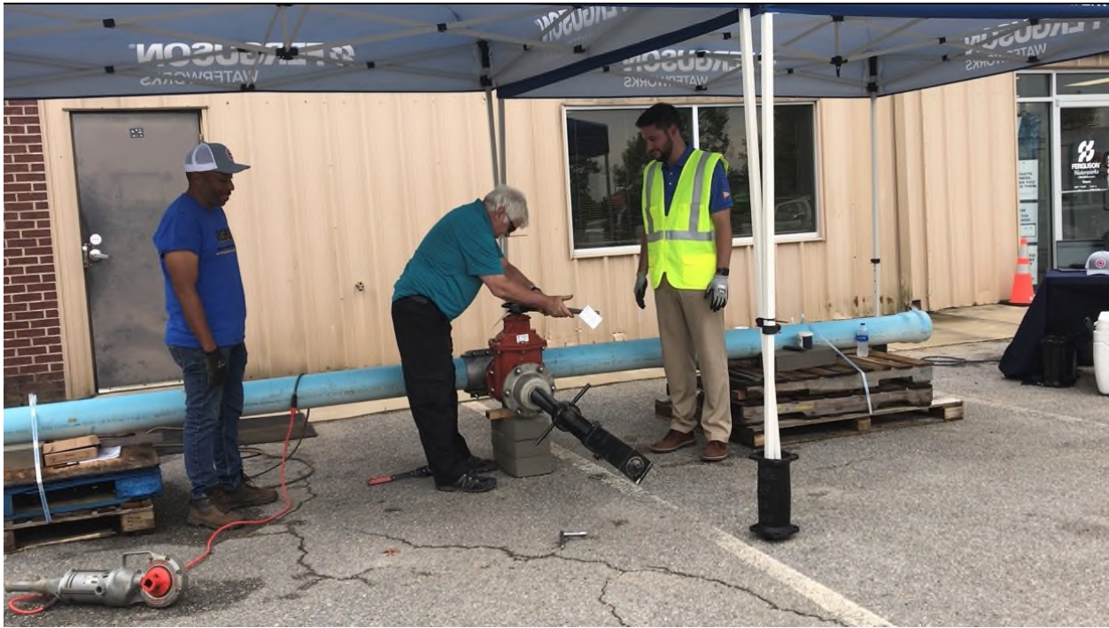
Left to right: Todd Corley, Corley Construction, Pat Ferguson, Ferguson Waterworks & Hamilton Cox, Ferguson Waterworks
