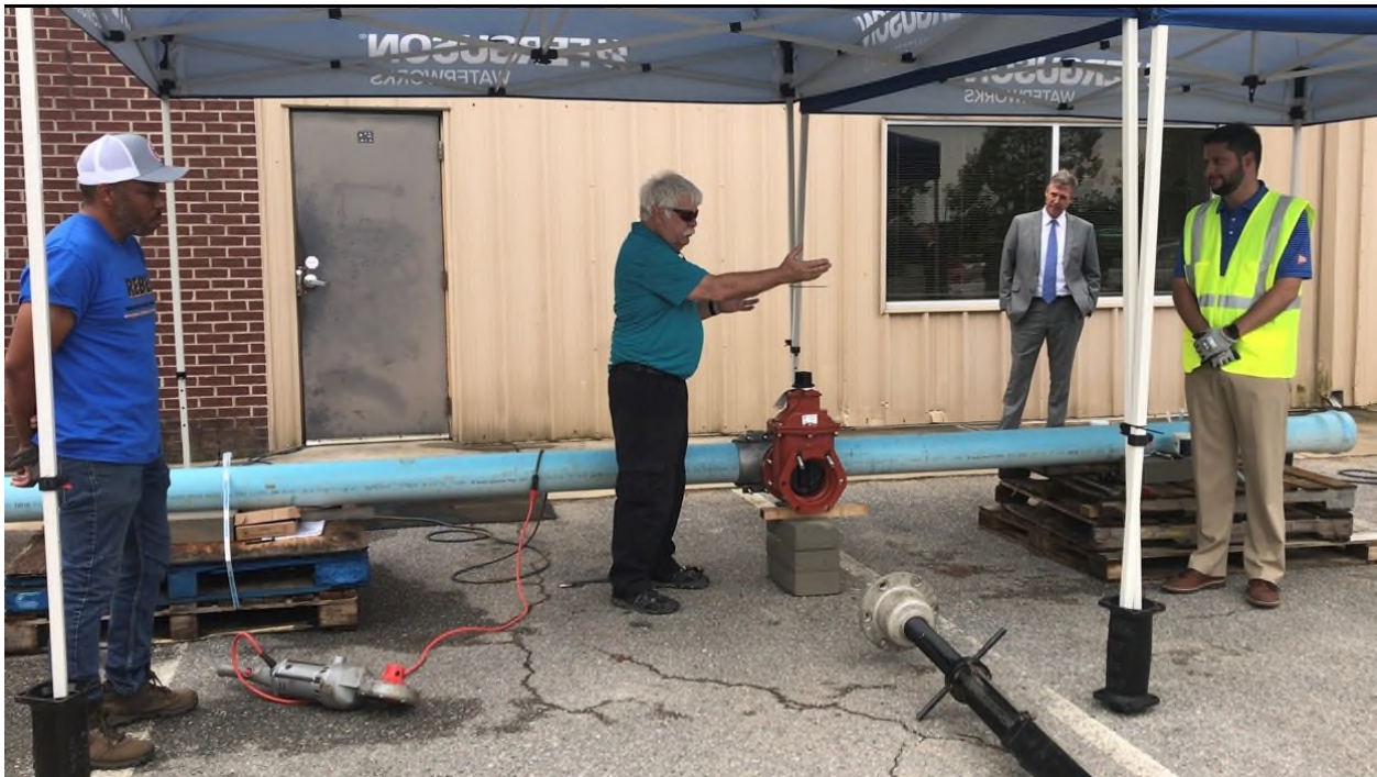
Left to right: Todd Corley, Corley Construction, Pat Ferguson, Ferguson Waterworks, Mayor Daniel Rickenmann, Hamilton Cox, Ferguson Waterworks
